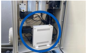
Demand control (centralized controller) IMP Atsugi
