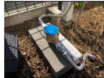
Install sub-meters on automatic sprinklers and monitor water consumption in more detail to save water
