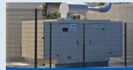
Emergency power generator
